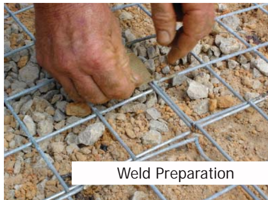
Unprepared Thermit Weld
